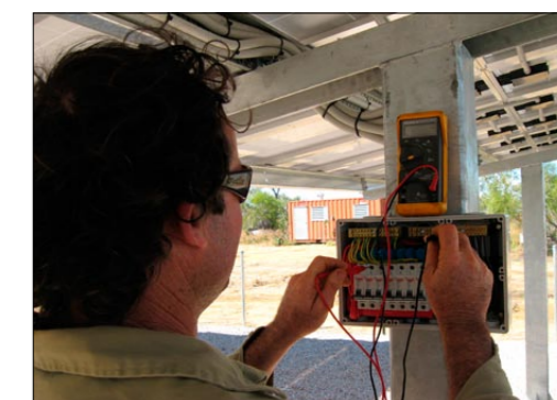
Robert Gulberti of Gully's Electrical testing PV string voltages on an array in the Kimberley, WA
