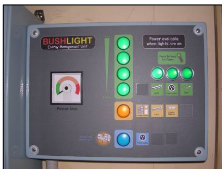
Energy Management Unit
