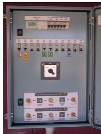
Alyuen's switchboard box
