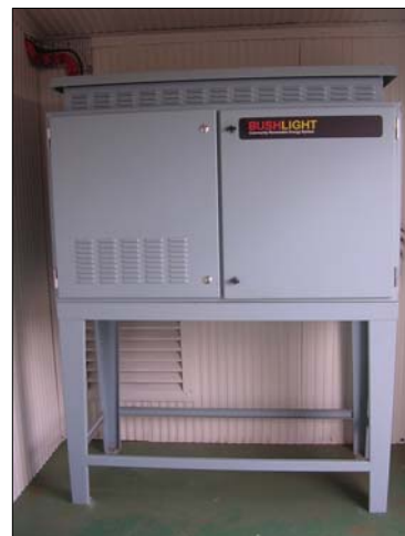
Mt Eaglebeak System Enclosure
