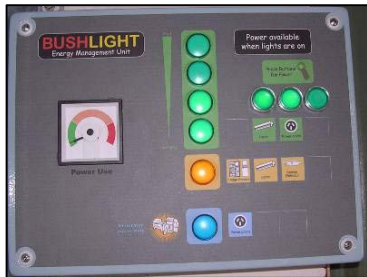
Energy Management Meter
