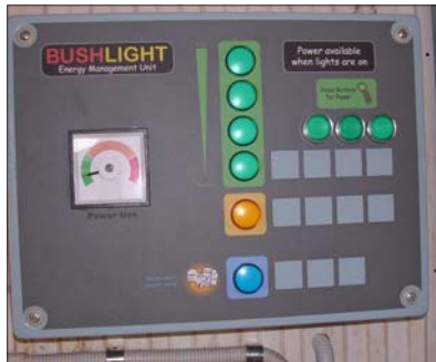
Energy Meter Unit
