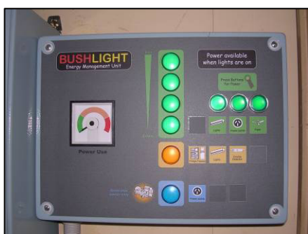
Energy Management Unit
